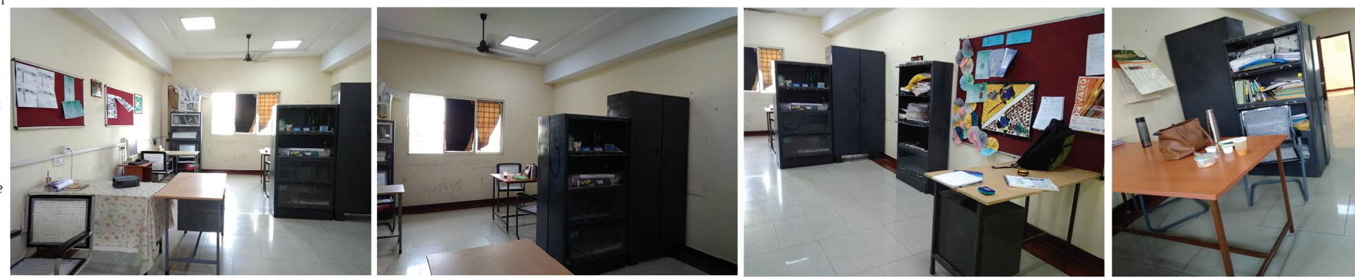
Provision of electrical points are only on one side of the room. Wiring is left unattended which is considered to be unsafe Provision of Lockers are improper and insufficient Beams and columns are not visually appealing. No proper dining space provided
